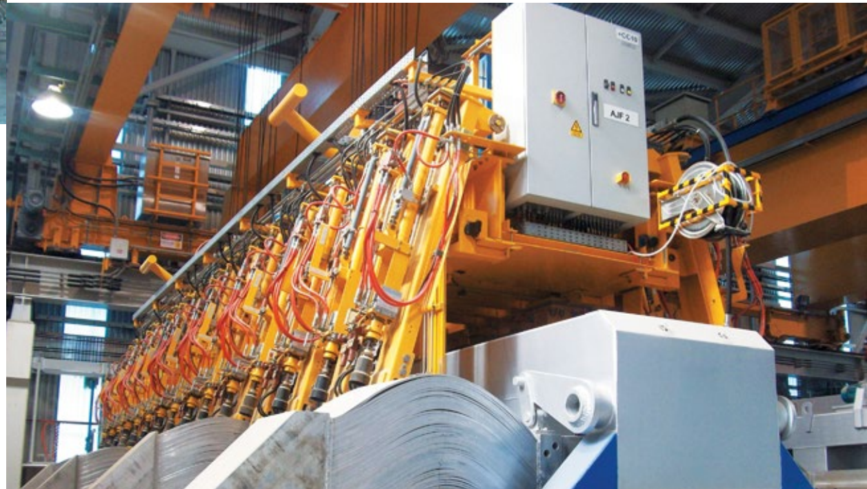
Pot Tending Machine; Anode Jacking Frame
