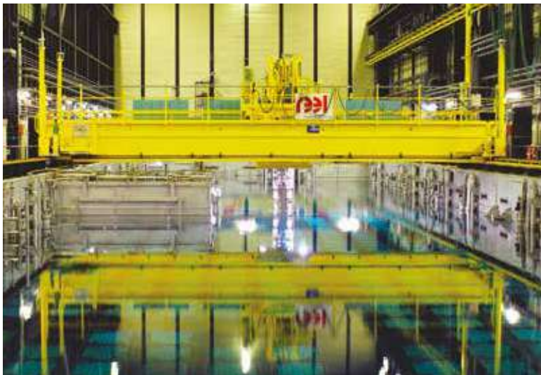
Spent Fuel Crane in La Hague
